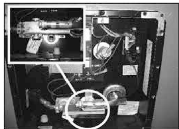
Fig 1: Water heater drain plug
